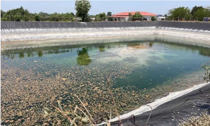
09. Water Storage pond 1: 10 million ltr
